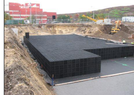
Underground detention tank Source: www.webtecgeos.com
