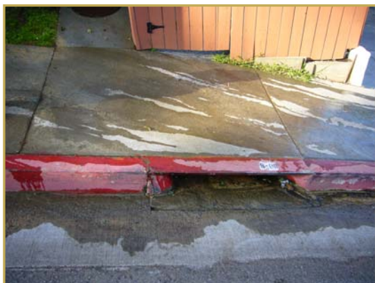
Irrigation runoff—water intended for landscape is now going down the storm drain.
