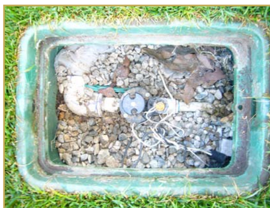
In-line irrigation valve installed underground inside a protective box.
