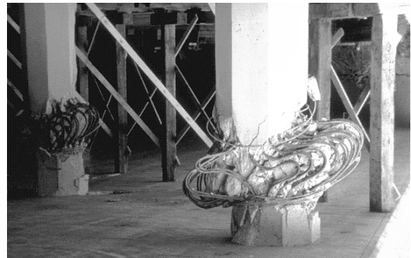
Failed Support Columns - Northridge
